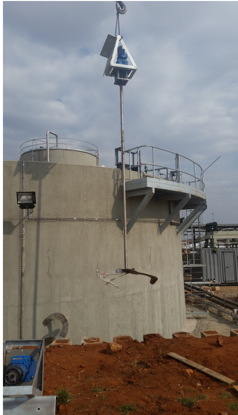
Anti-ragging propeller and shaft installation at effluent treatment
