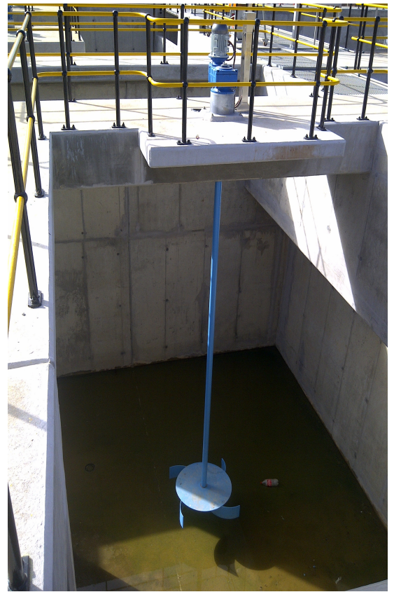
Top-entry mixing unit at a municipal waste-water
