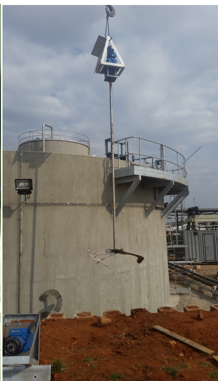
Anti-ragging propeller and shaft installation at effluent treatment plant
