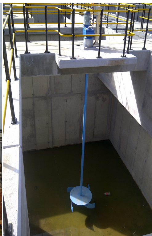
Top entry mixing unit at water- treatment plant
