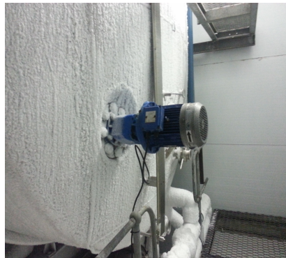
Side-entry mixer on a 50 000L horizontal cold-stabilisation tank, running at - 4C
