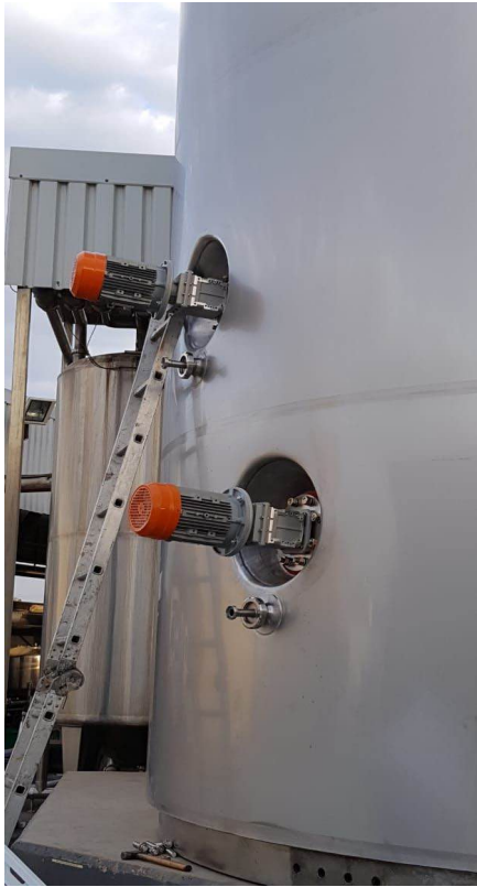
Twin Side-entry mixer installation a higher mixing turn-over rate
